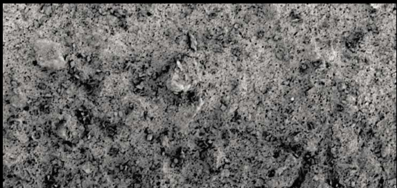
Grout in the tiled area rough, porous
